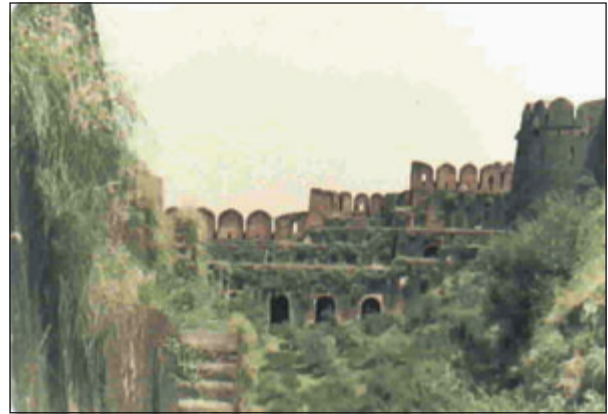
Fig. 1. The dilapidated Rohtas Fort buildings, Jhelum River valley, Punjab, Pakistan. Hemidactylus flaviviridis are collected from roofed parts, while from exposed parts of the buildings H. persicus , H. brookii , Cyrtopodion montiumsalsorum , and rarely C. scabrum were picked up.
